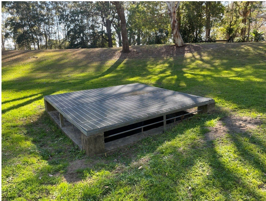
Figure 2-10: Example of Raised Grated Letter Box Pit Inlet at Detention Basin on Langford Drive near Arunta Avenue
