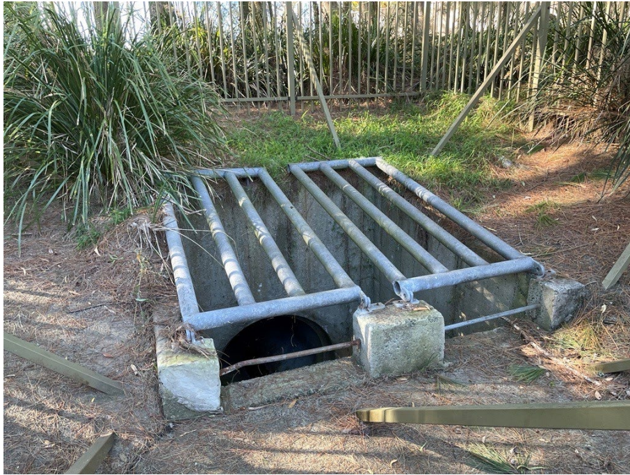
Figure 2-11: Grated Inlet at Detention Basin on Langford Drive near Arunta Avenue
