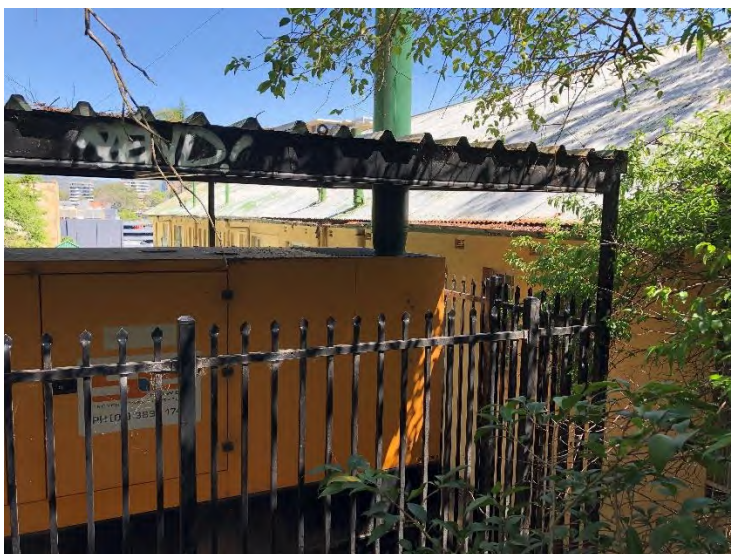
Photograph 5: Existing on site generator
