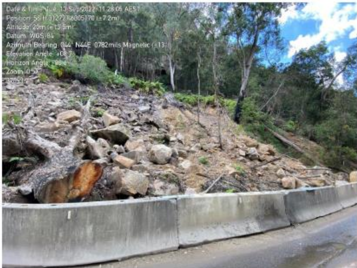
Figure 1-3 views of the damaged roadway looking south east
