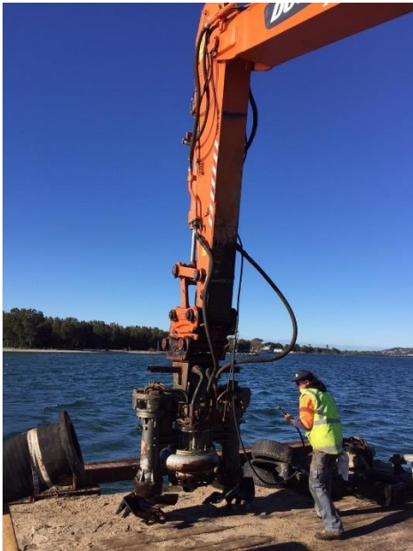
Photo 1 Submersible pump and associated cutters
